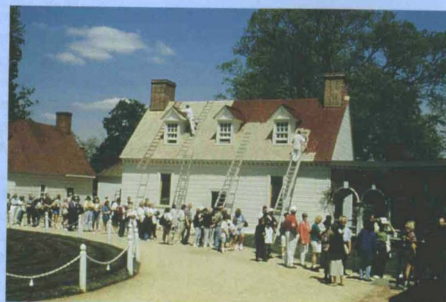
The newly repaired and resingled cypress roof of the Servants' Hall was eventually painted.
