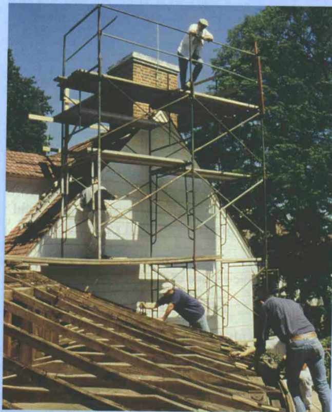
The north colonnade, which connects the Servants' Hall with the Mount Vernon Mansion, saw the replacement of shingles and sub-structure repairs.
