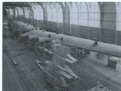
This view shows the wings under construction. Their span was longer than a football field.
