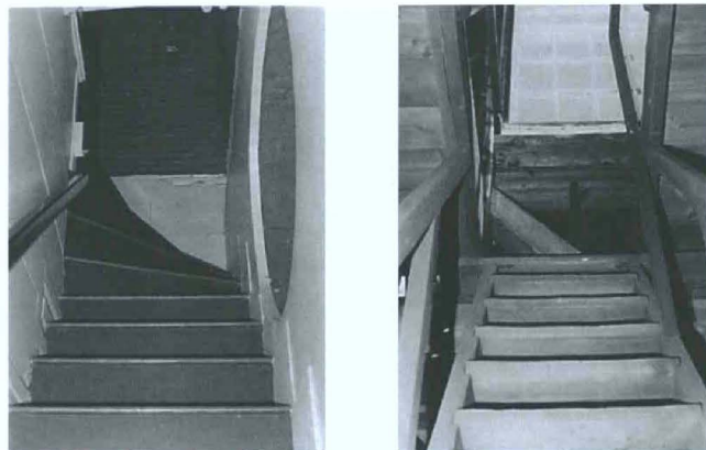
These photos taken at the Old North Church dramatically illustrate the precarious path taken by those who hung the lanterns in the Old North Church. Shown at the left are steps to the first landing in the steeple, while that at the right shows the ladder steps that lead to the highest window in the steeple. (Photos taken by Robert Newman Sheets in 1980. Property of The Newman Family Society.)
